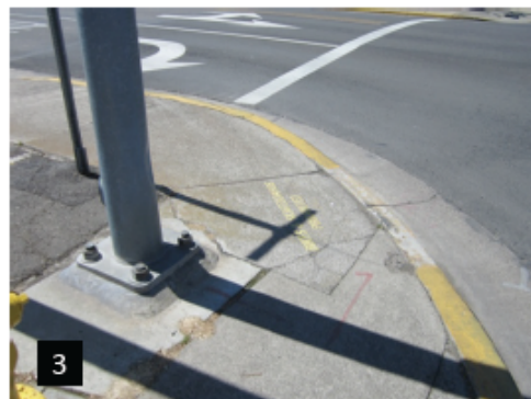
The series of pictures above illustrates current sidewalk conditions on E. Pine Street. [1] sidewalk in disrepair [2] obstructions in the traveled way [3] poor curb ramp design with an obstructed landing
