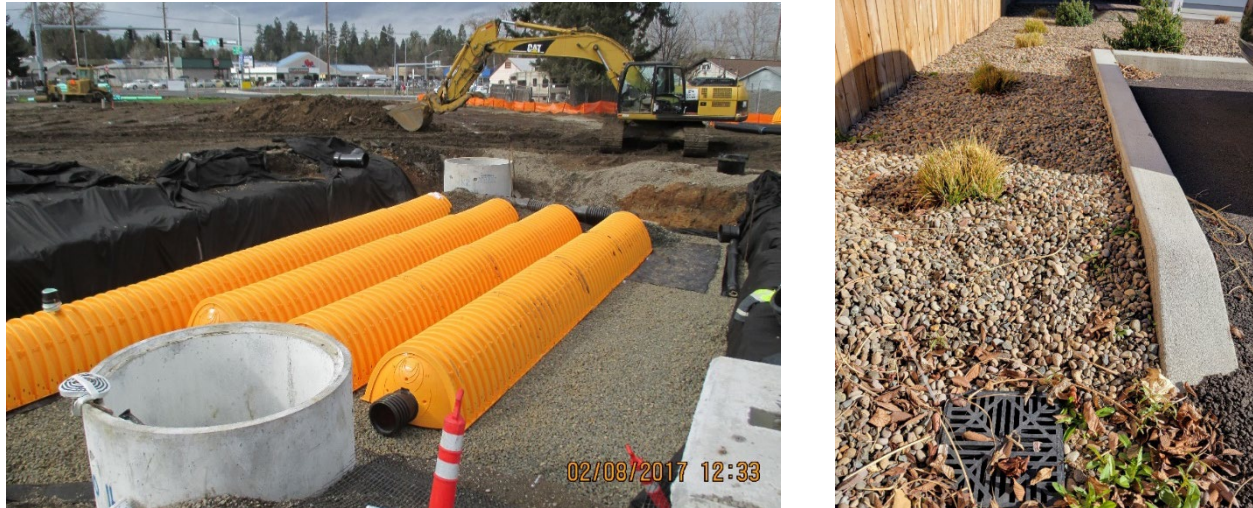
Figure 4.4. Underground chambers (let) are one example of underground Retention when designed to fully infiltrate the Retention storm. Underground Retention can also be designed under a landscape area (right).
