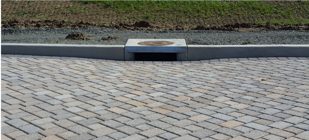
Figure 4.3. Permeable Pavers intercept rainfall and infiltrate it into the ground, the catch basin will only receive runoff from large storm events.
