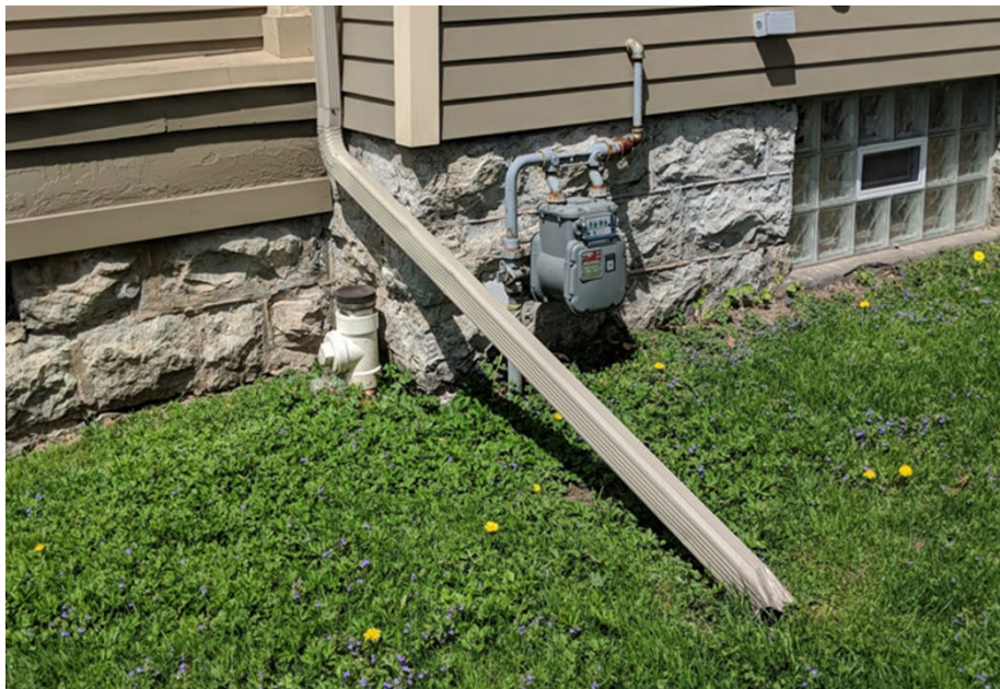
Figure 4.9. Disconnected Downspout (Picture Courtesy Rain Check Buffalo )
