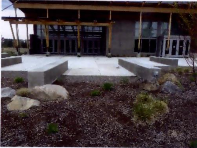
Figure 4.9. Example of sheet flow from a patio to a newly installed vegetated filter strip.
