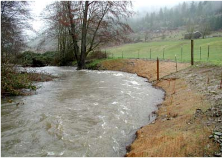
Figure 16.—Erosion-control matting was used on this section of Thompson Creek, in Jackson County, after a steep, eroding bank was graded back to a more desirable angle, exposing bare soil. The site was revegetated with willow cuttings (visible as stakes in the fabric) and grass. Photo courtesy of Applegate River Watershed Council.
