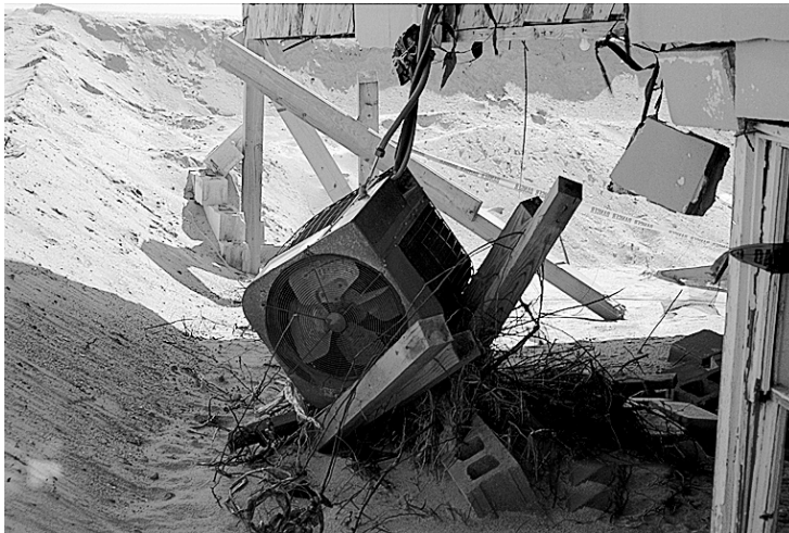
Figure 1.2.1A: Electric heat pump dislocated from its shattered wooden stand by velocity flow in a coastal area
