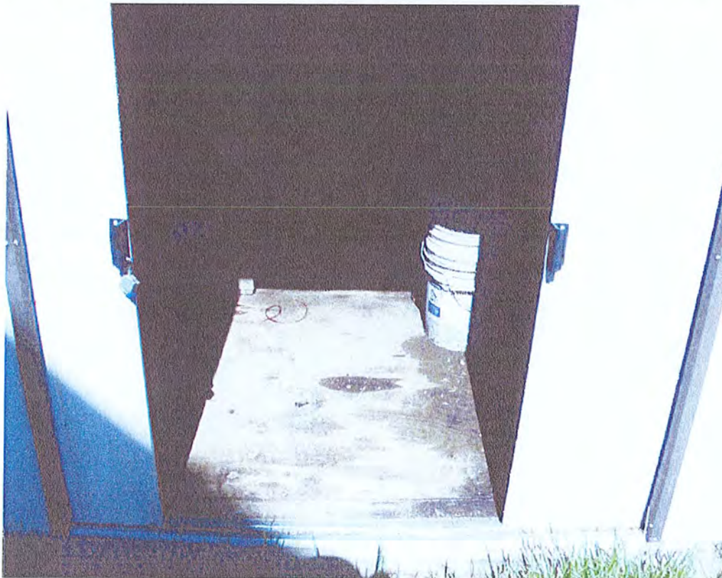
Photograph 14. Stains from petroleum products were observed on the floor of the small shed.
