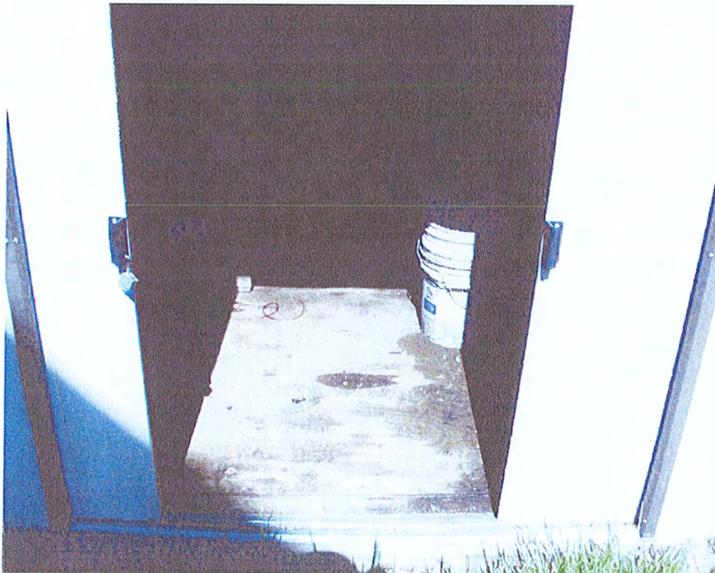
Photograph 14. Stains from petroleum products were observed on the floor of the small shed.
