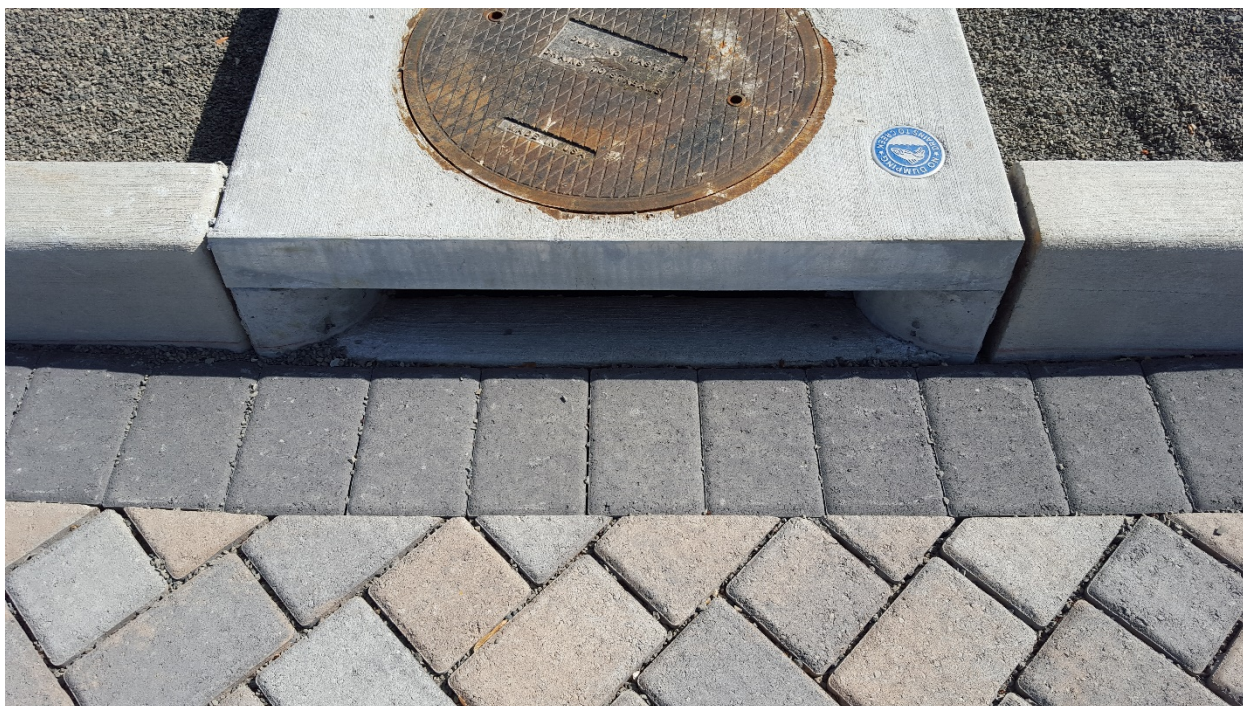
Figure 4.3. Porous pavers intercept rainfall and infiltrate it into the ground, the catch basin will only receive runoff from large storm events.
