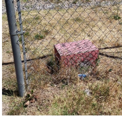
Water valve located at each field.
