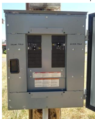
Field light exterior circuit breaker.
