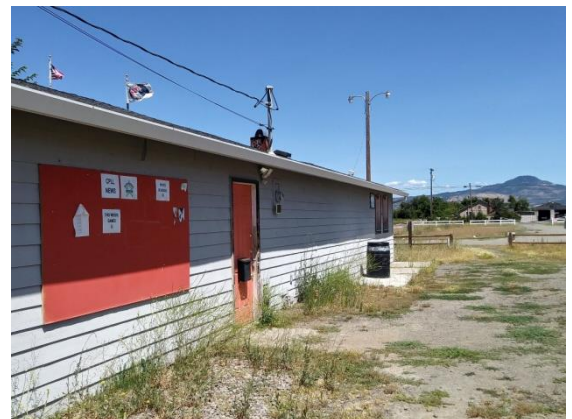
Concession stand electricity.
