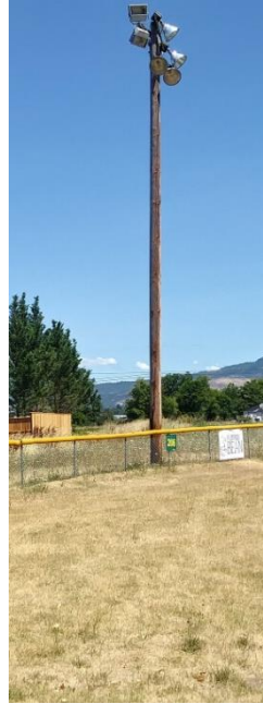
Utility pole with field light.
