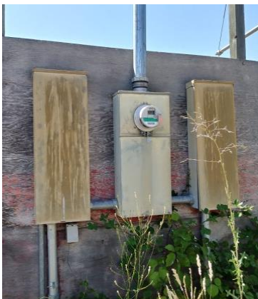
Exterior meter on site.
