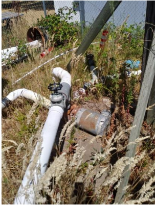
Pump outside storage building.
